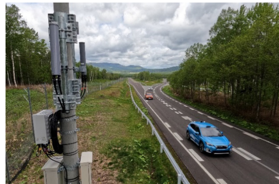
Local 5G equipment installed at the circuit
