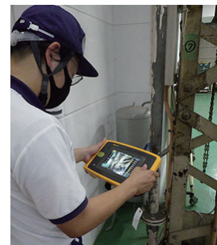
Air leak investigation
