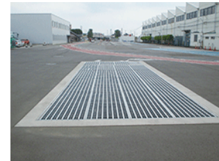
Flood prevention measure (drainage grid) (Utsunomiya Plant)
